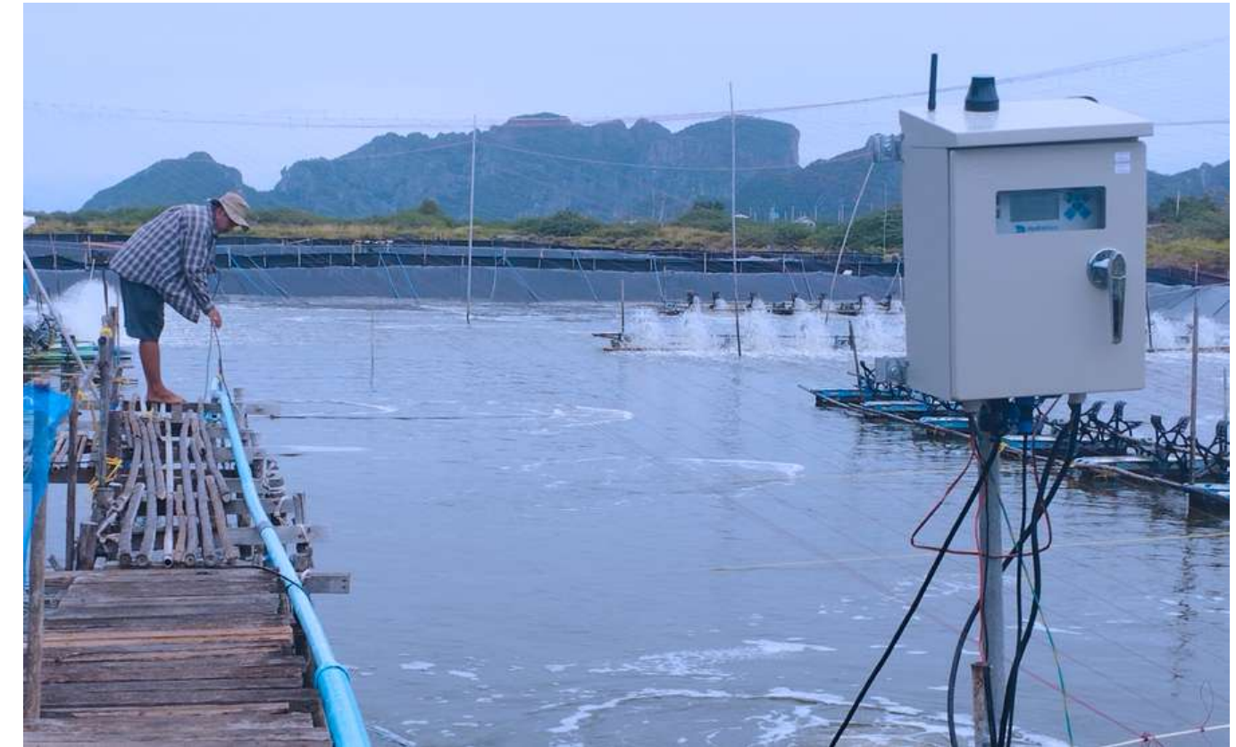
Hydroneo aerators to enhance water quality
